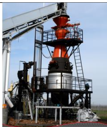
Phoenix Energy power plant produces 500 kWe and biochar from residues in Merced, California. www.phoenixenergy.net
